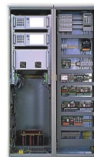
Electrical control panel
